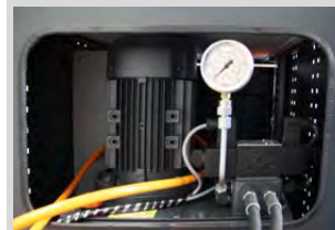
Dual-circuit hydraulic unit in cabinet base
